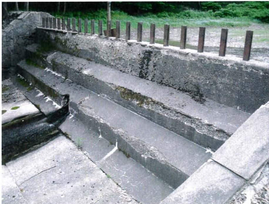
Photograph No. 8: Weathering and erosion of Silver Creek Detention Basin Dam.
