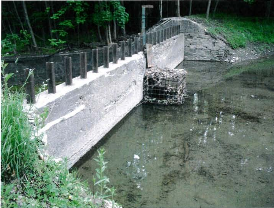
Photograph No. 13: Upstream face of dam's spillway section. Structural crack noted in foreground above water line.
