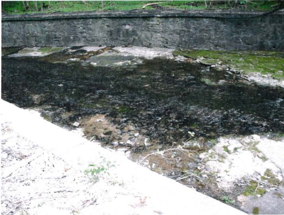
Photograph No. 9: Weathering and deterioration of downstream channel.
